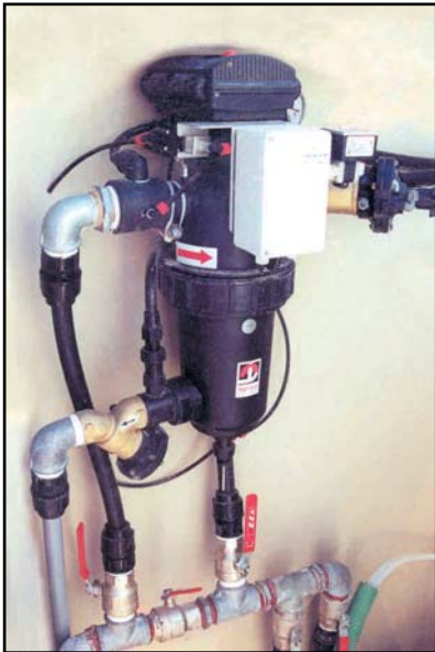
Communal housing, intake water - ISRAEL
