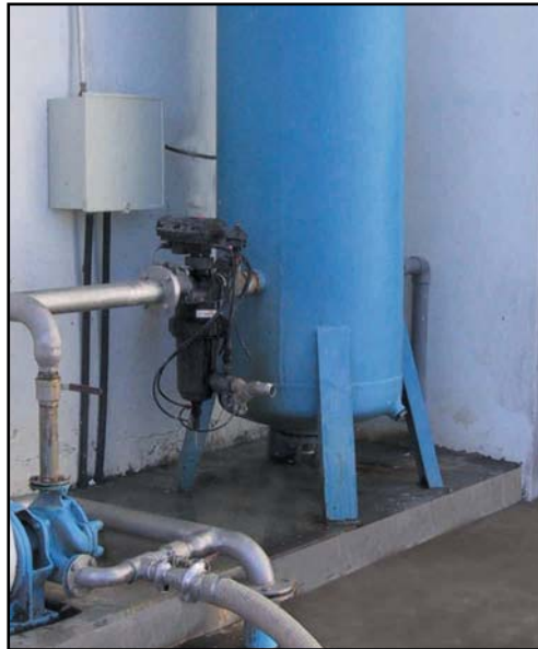
Intake water, prior to a softener at a winery - SOUTH AFRICA
