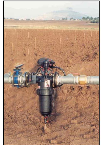
Drip irrigation of reclaimed water - ISRAEL
